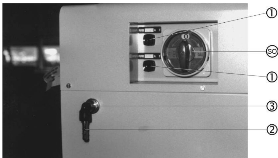
Fig. 32 Main Switch and Fuses
