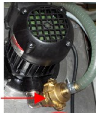
A Pump outlet
